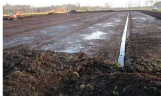
8 Precise top soil removal and installation of irrigation ditches for the Sphagnum farm (Photo: J.-U. Holthuis)
