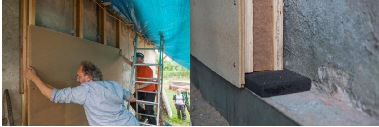
Fixing soft-fibre insulation tiles at the wall for preparing the „blow in test“ (left) and bottom construction details (right)
